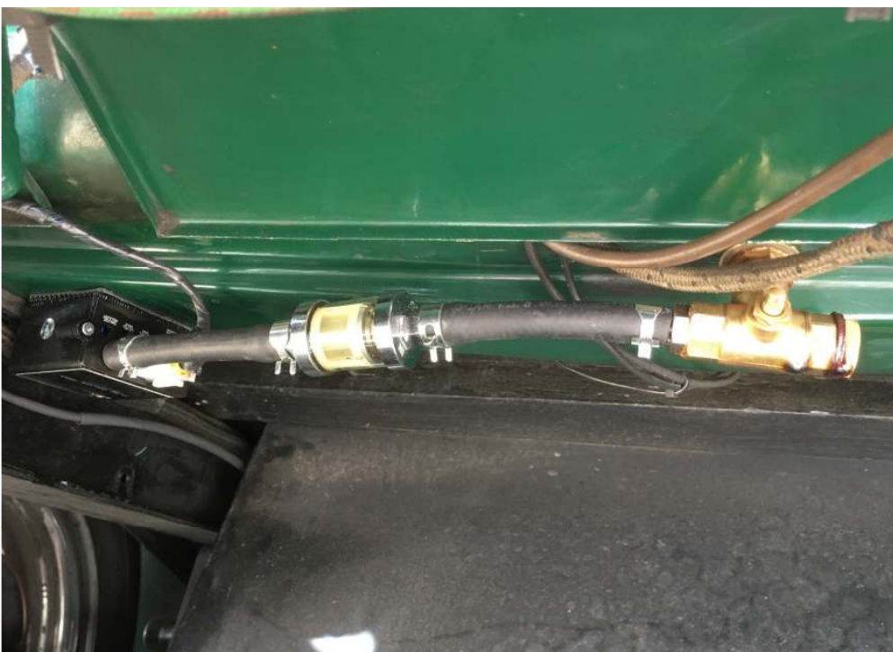
Photo 4 - Installation with filter. The handle on the ball valve was removed on this installation.
